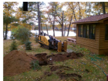
Geothermal heat pumps rely on energy of the ground to move heat into and out of a building, providing winter heating and summer cooling.
