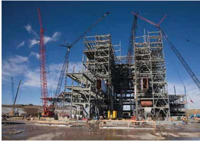
Dry Fork Station, a coal-based electric generation power plant owned by Basin Electric Power Cooperative and the Wyoming Municipal Power Agency, came online in August 2011. Located six miles north of Gillette, WY, the $1.35-billion Dry Fork Station is Wyoming's newest coal-based plant. The new plant helps Basin Electric meet the power needs of its 135 member cooperatives.
