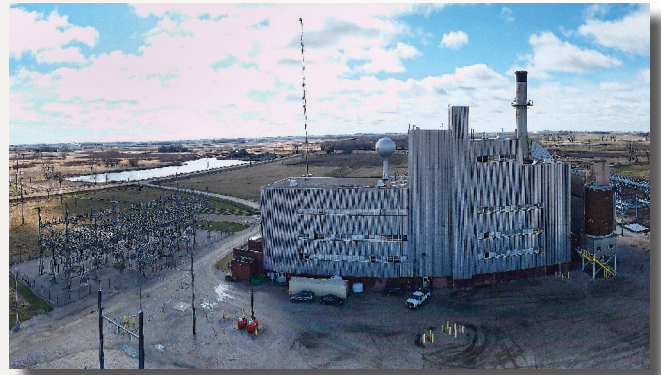
Corn Belt Power Cooperative's Wisdom 2 Substation located in Spencer, Iowa
